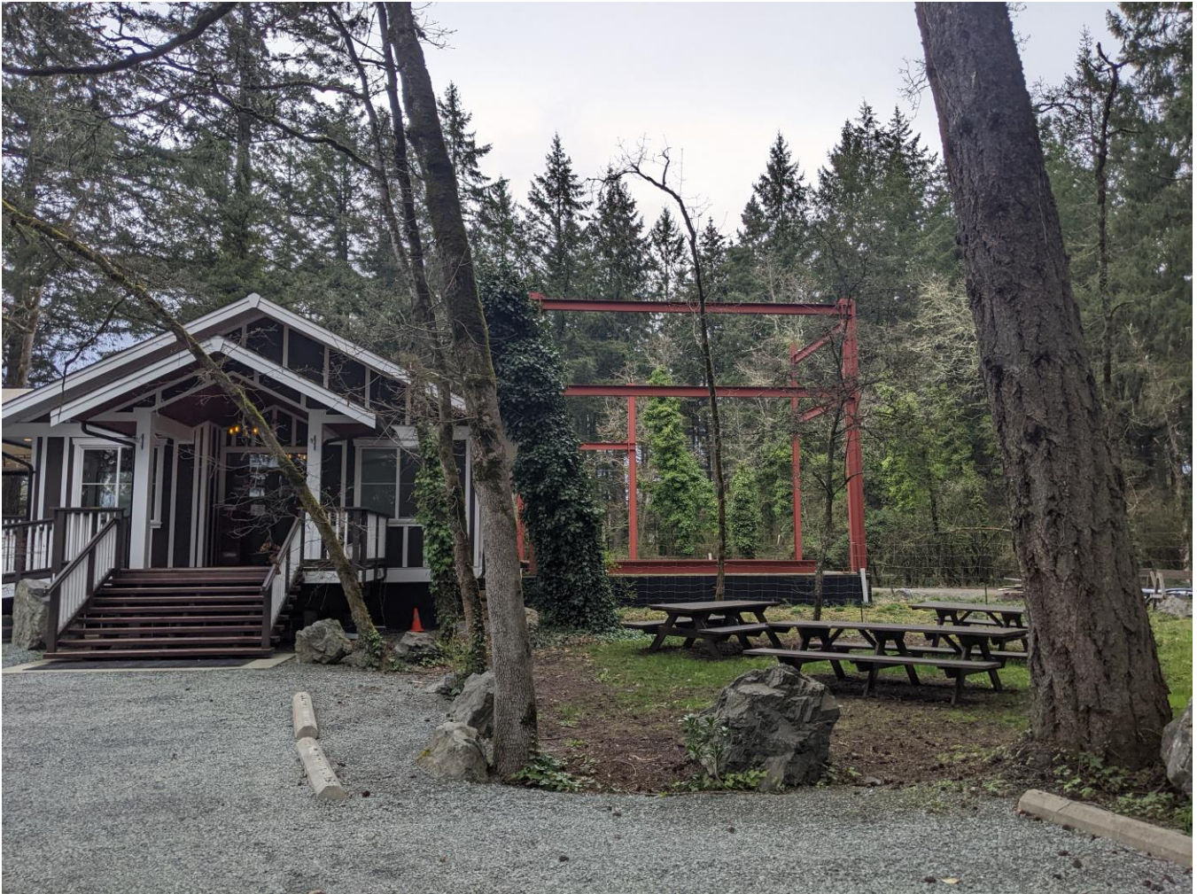
Photo 6 & 7 – Rear and side view of the partially constructed cold storage building addition.
