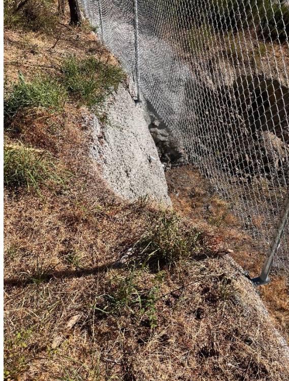
Photo 3 - Example of the gap at the base of the fence.
