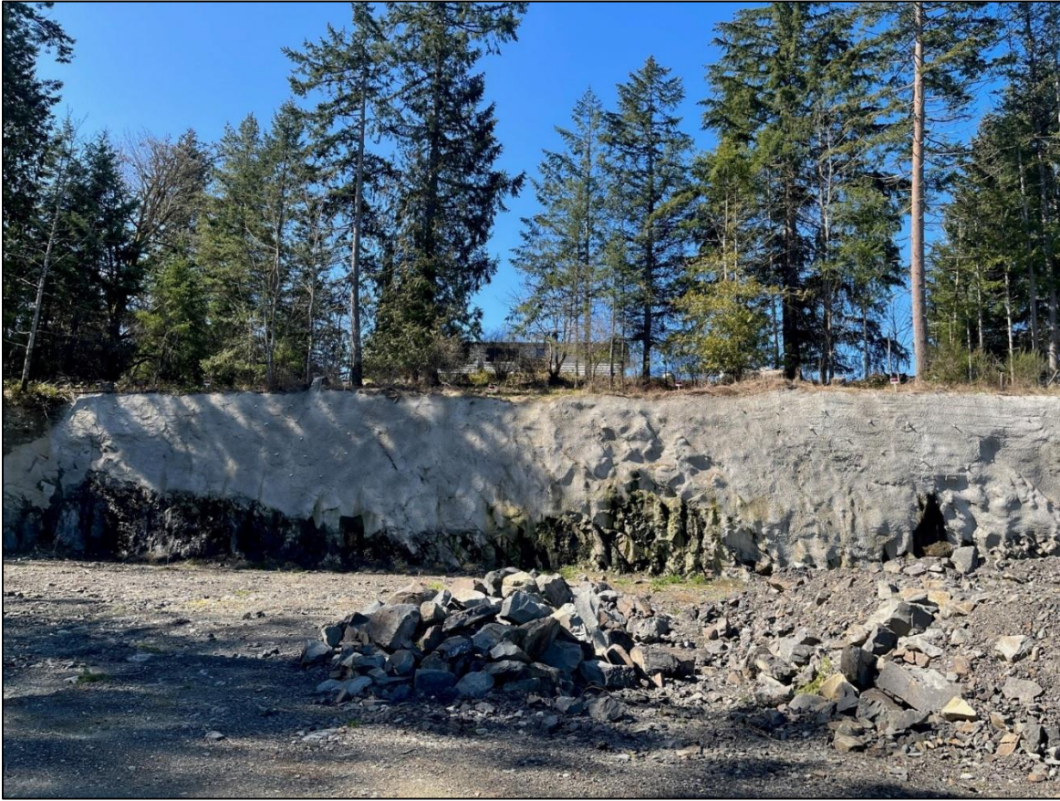
Photo 1 - Unprotected embankment, April 2023
