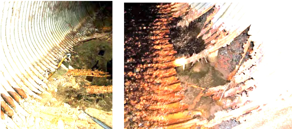
Figure 10 Examples of failing Corrugated Metal Pipe (CMP) culverts.
