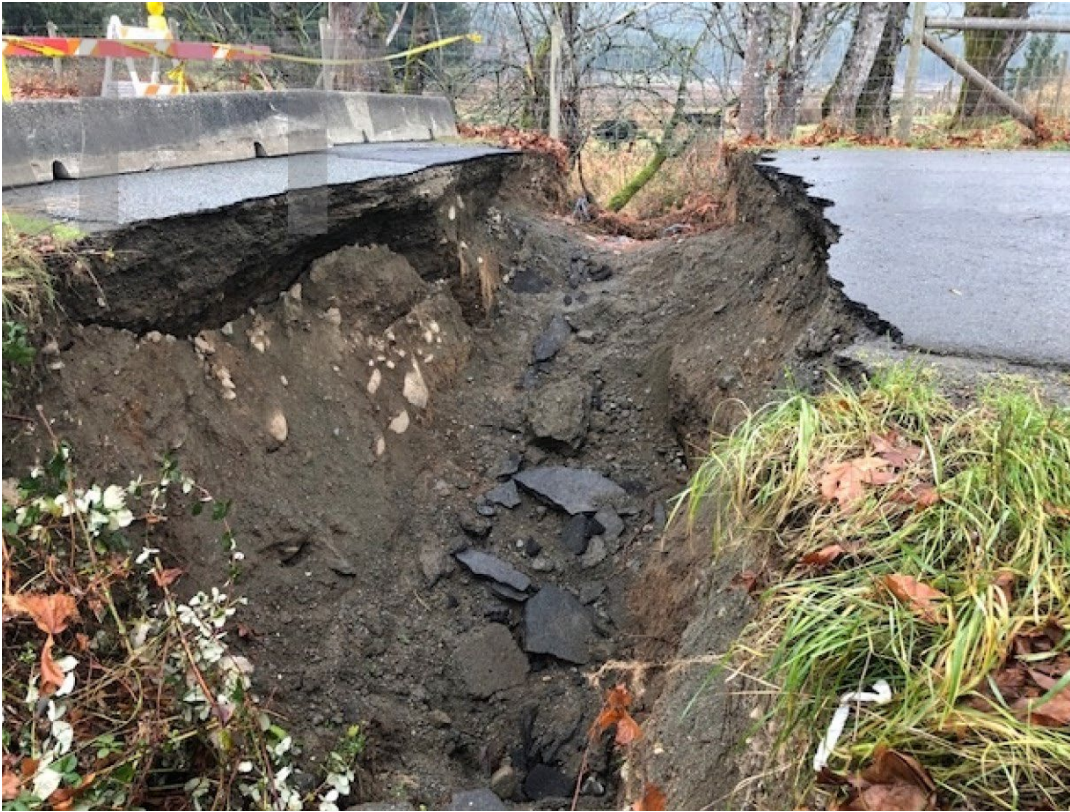
Figure 11 Section of Mays Rd where flow diverted around a culvert ultimately resulting in the washout of the road.
