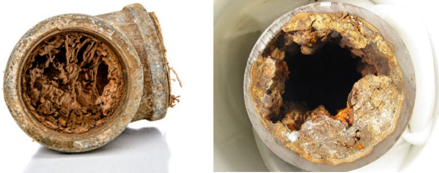
Figure 9 Examples of tuberculated cast iron pipe.
