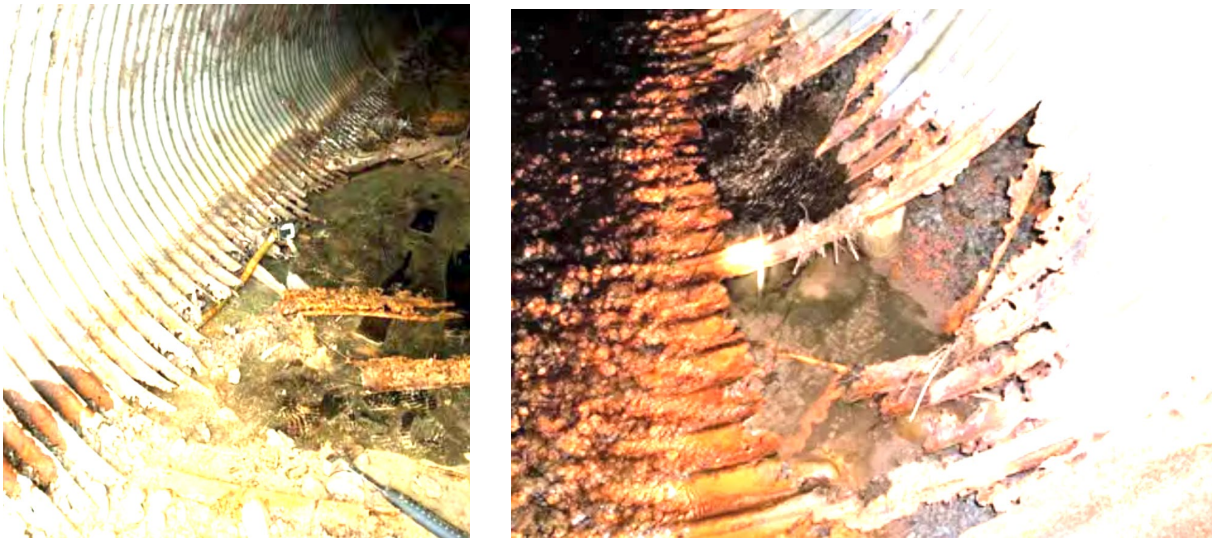
Figure 5 Examples of failing Corrugated Metal Pipe (CMP) culverts.
