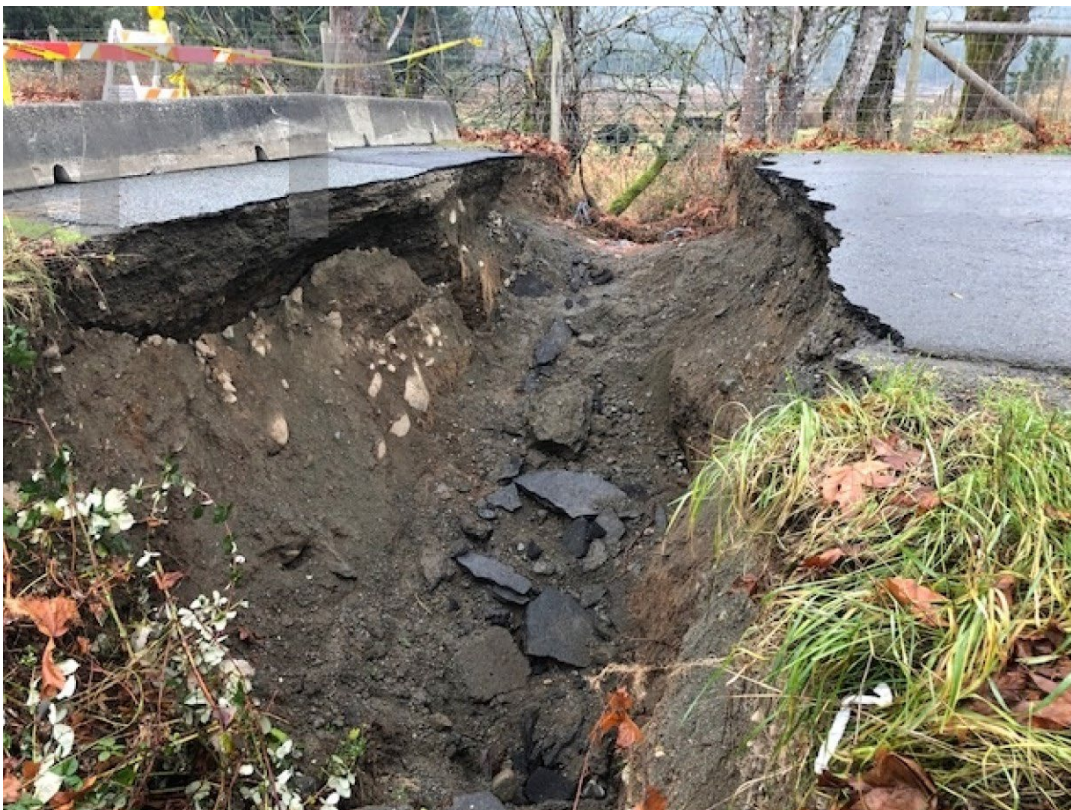
Figure 6 Section of Mays Rd where flow diverted around a culvert ultimately resulting in the washout of the road.
