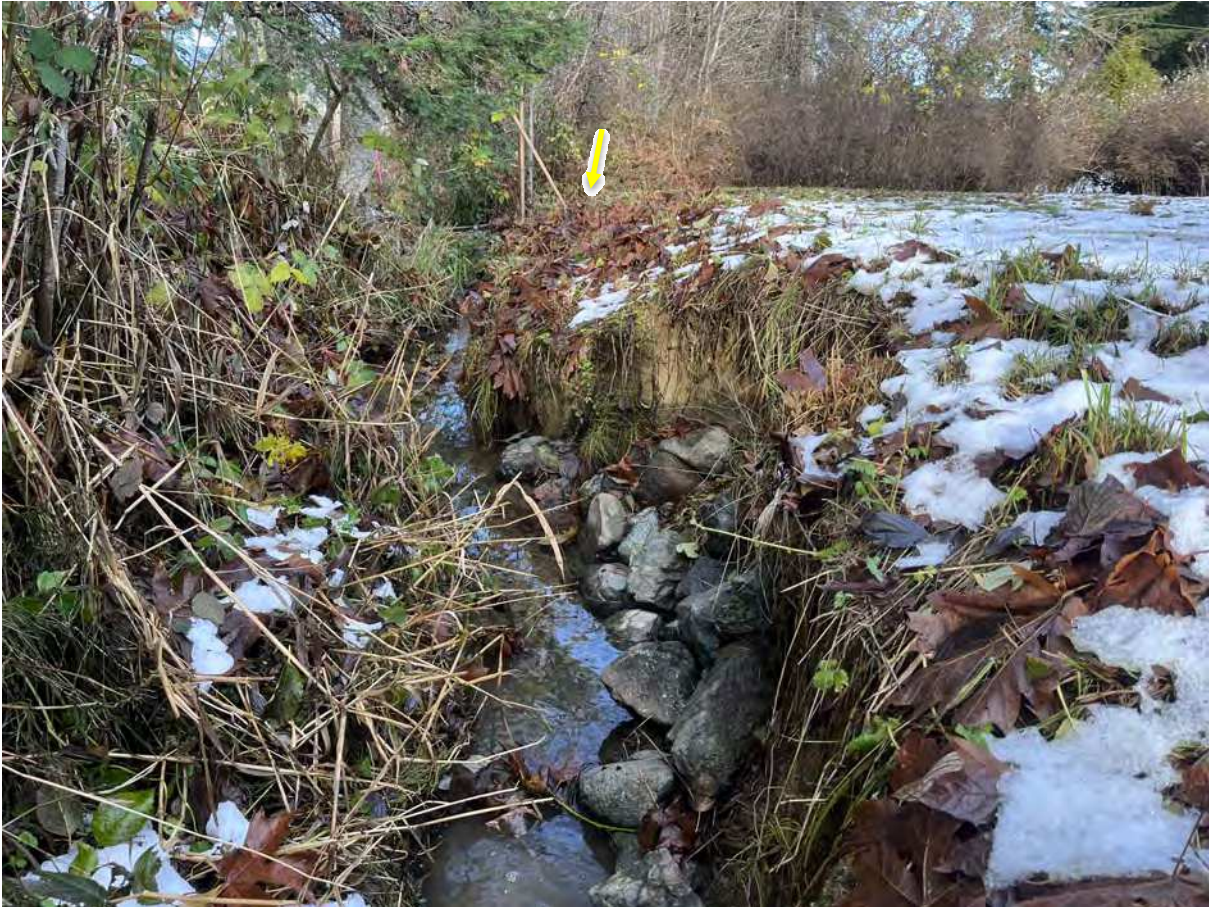
Figure 19. Looking downstream along Ditch 1 (1937 Maple Bay Road). Note the turf lawn on the east side of the channel, the moderate channel entrenchment, shrub understory on west bank, and the rock armouring placed in the channel to try and arrest bank sloughing on the east side. The yellow arrow indicates the property boundary between 1935 and 1937 Maple Bay Road (Figure 10).
