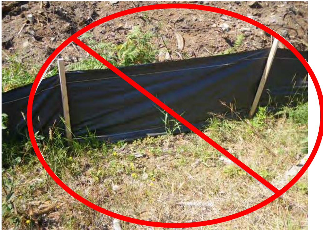
Figure 2. An example of an incorrectly installed silt fence. The posts are on the correct side of the fence, but the tail is not buried at all. The coloured line along the edge of the fence is still clearly visible, and it is less than 5 cm from the bottom. This fence will not control runoff.
