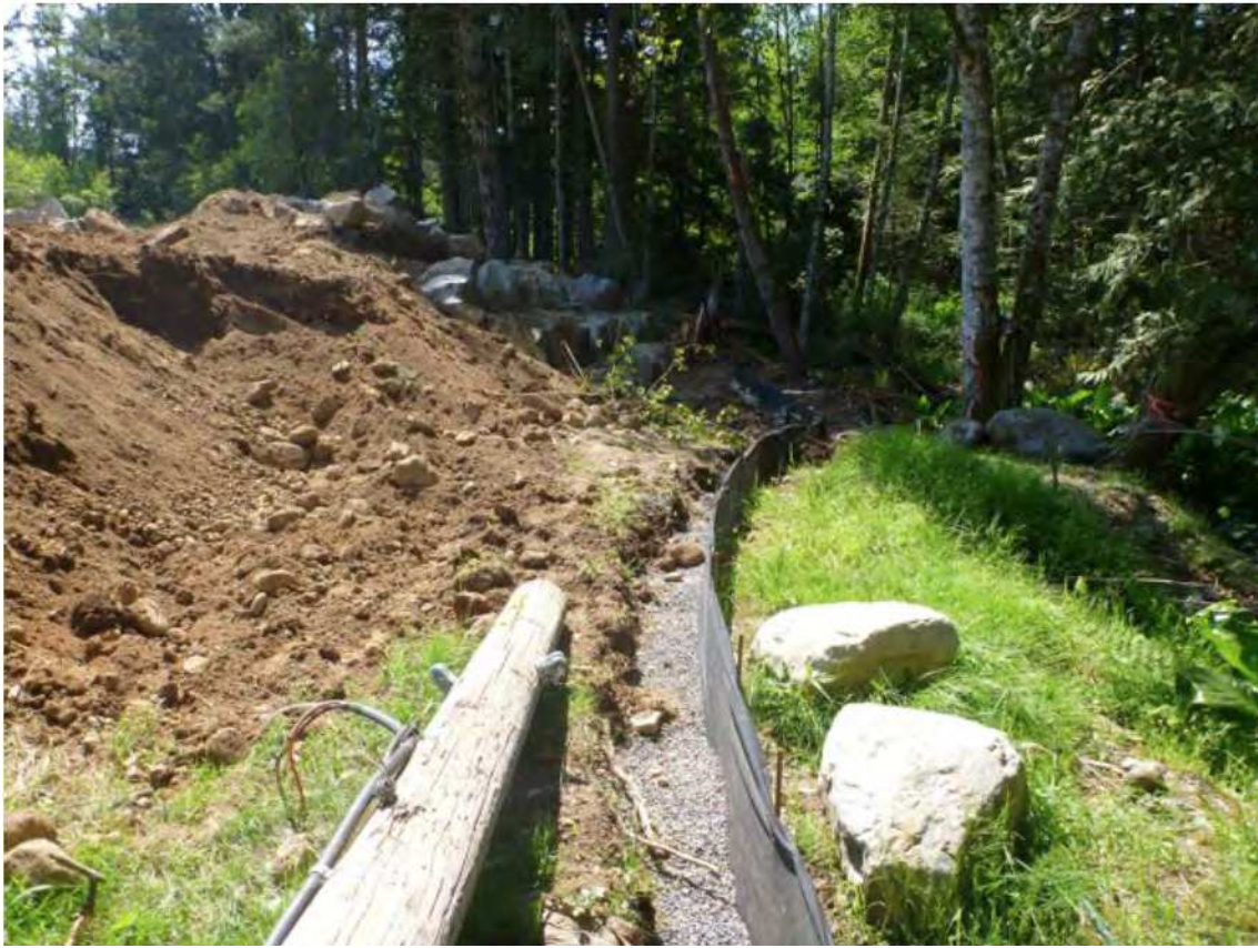
Figure 5. An example of a silt fences installed with filtering pea gravel trench.
