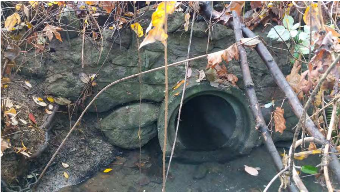
Figure 27. The outlet of the culvert under Maple Bay Road and its shallow plunge pool; the shallow plunge pool indicates there are typically insufficient stormwater volumes to scour a deep plunge pool at the outlet.
