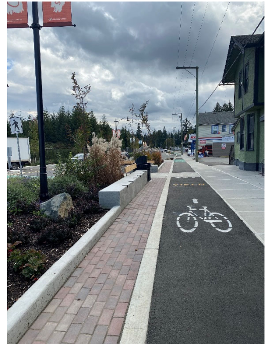
Uni-directional bike lanes were implemented along a segment of Chemainus Road (Henry Road to Victoria Street) in 2020, making these facilities the first protected bicycle lanes in North Cowichan.
