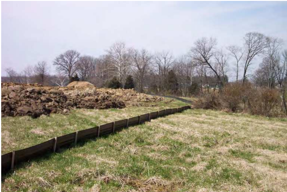
Figure 1. An example of a properly installed silt fence. The fence is tight and the posts are on the downstream (downhill) side. There are no gaps under the fence.
