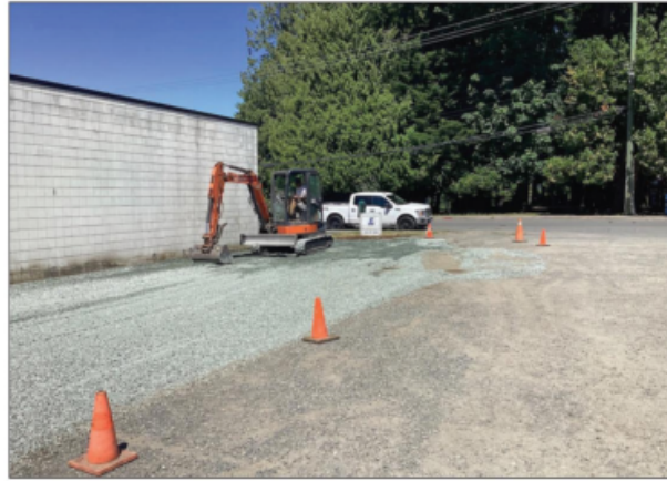
Work has begun to prepare the vacant lot at 9800 Willow St. to become a community garden. (Photo courtesy of Kate Marsh)
