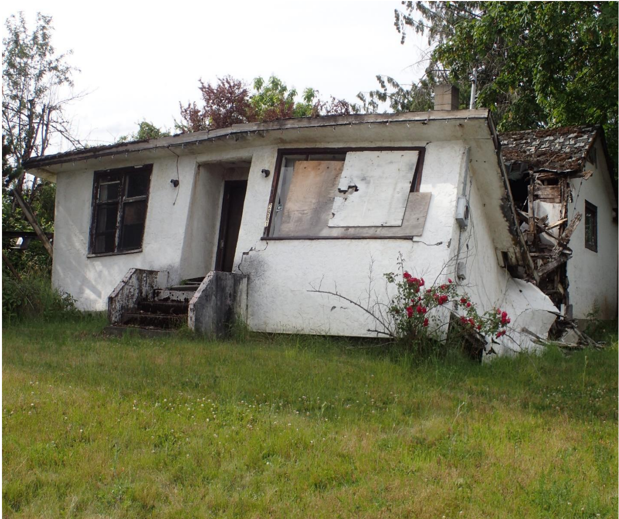
Images – hazardous structure 2961 Sherman Road
