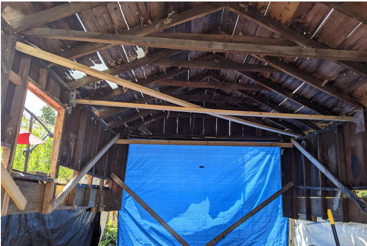
- Interior view, the building was temporarily braced in order to keep it from collapsing due to decay.
